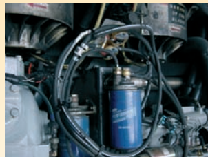
Carrier Diesel Generator
